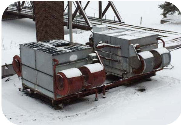
Chiller Units (caulk) Mech. Room Roof
