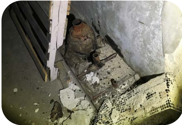
Pipe Mastic (Coolers)
