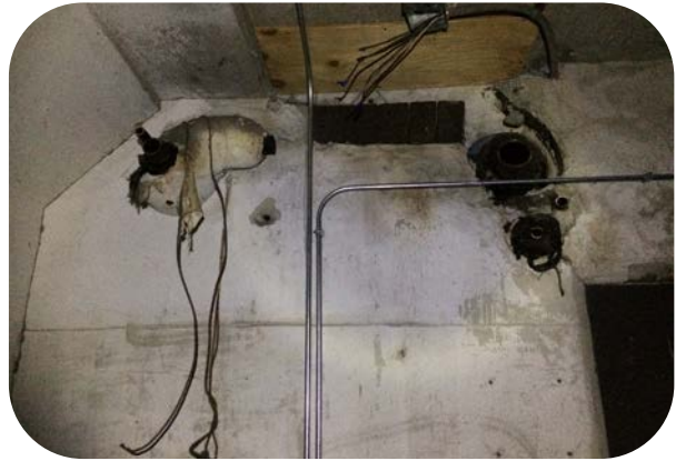
Muddied Fittings & Pipe Mastic (Coolers)
