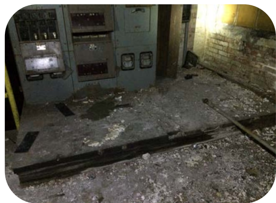
Transite Floor Panel (Mech. Bldg.)
