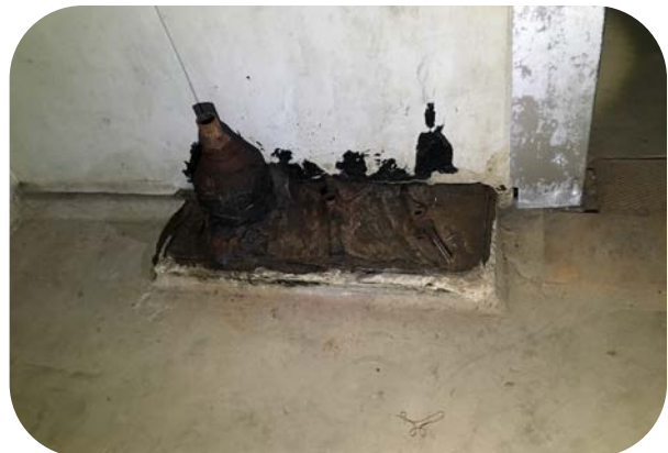
Pipe Mastic (Coolers)
